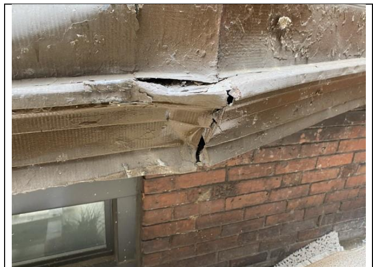
54. Typical cracking in rear bay window frame.
