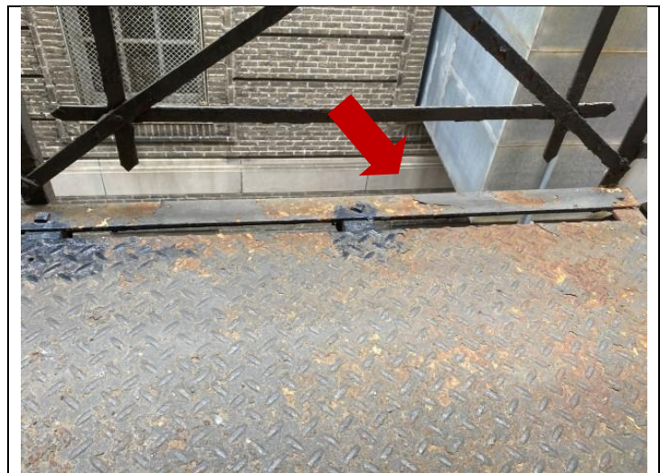
52. Typical corrosion found on egress balconies.
