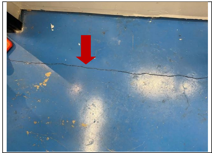
50. Concrete floor shrinkage cracking observed in the Amenity Building pool/spa mechanical space.
