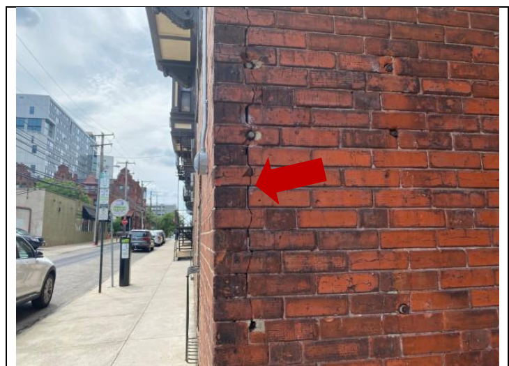
60. Vertical cracking at the rear of Building G.
