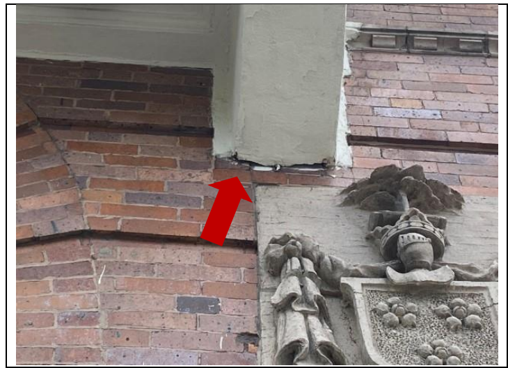
56. Typical void between diagonal balcony support and masonry wall on Buildings A and K.
