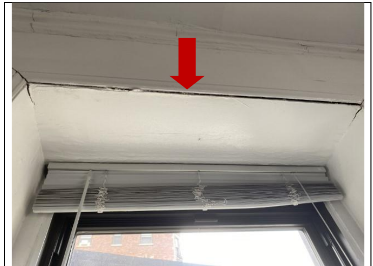
28. Large cracks in Building B window frame indicative of foundation settlement.
