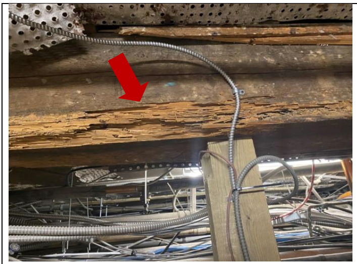
39. Termite-damaged wood beam in Building G and H basement.
