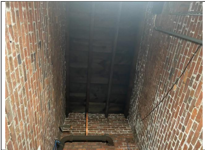
15. Typical exposed wood roof decking visible from the emergency egress stairwell in the apartment buildings.
