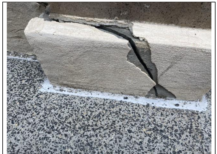
34. Large crack in decorative stonework base.
