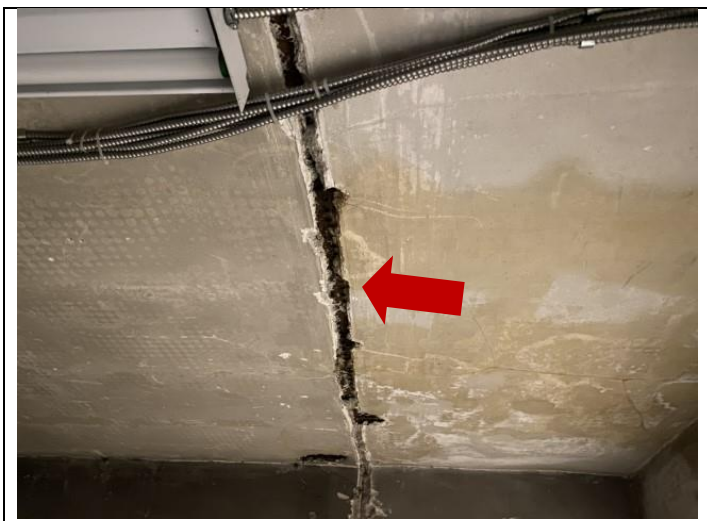
47. Cracking observed in Building D basement ceiling.
