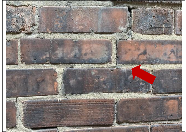
26. Stair-stepped cracking observed on Building B exterior wall.
