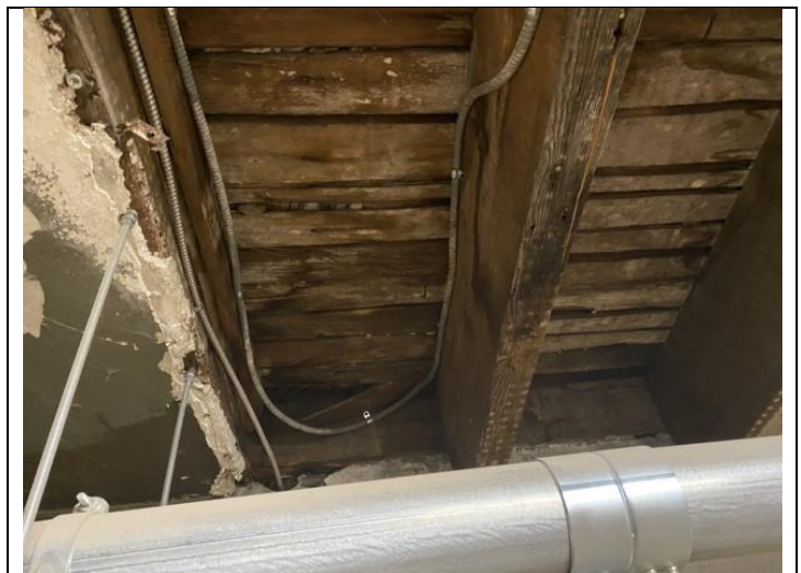
40. Water damaged and rotting wood floor joists visible in the Building G/H basement.
