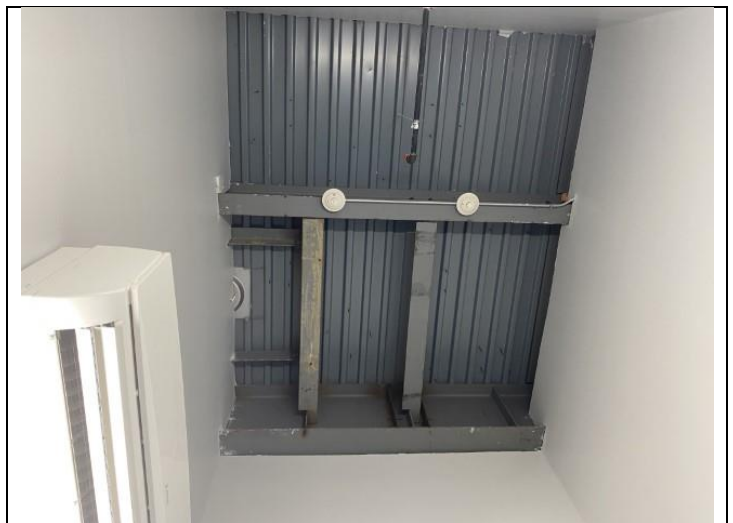
24. Exposed steel framing and metal roof deck visible from the Amenity Building pool mechanical room.
