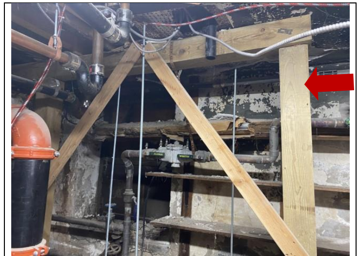
44. Retrofit wood columns and cross bracing that is not reflected on the structural bid set for Buildings G and H.
