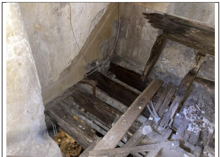
42. Rotted out wood plank flooring and joists in Buildings G/H basement.
