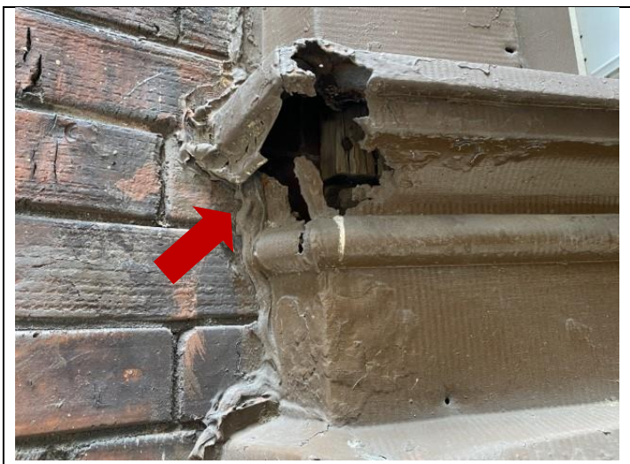
53. Typical void in rear bay window frame.
