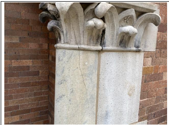
35. Hairline crack in decorative stonework column.
