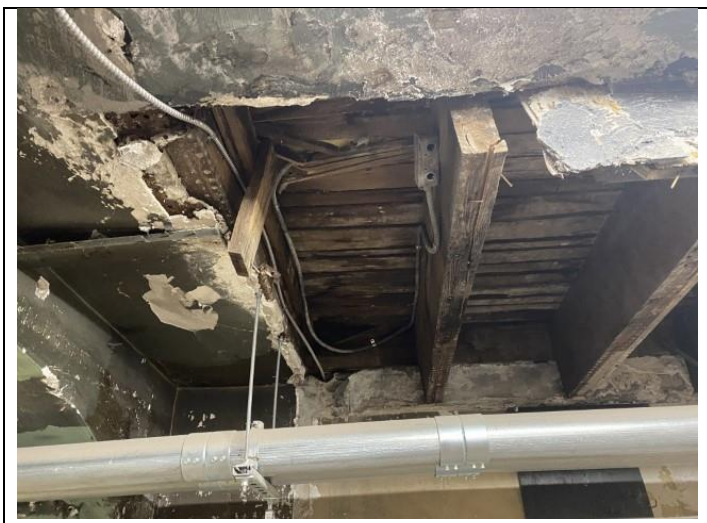
41. Snapped wood plank floor and joist visible from the Building G/H basement.
