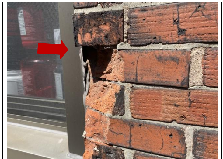
30. Typical section of spalling in exterior brick masonry.
