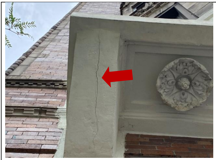
57. Hairline cracking observed on the left balcony on Building A.
