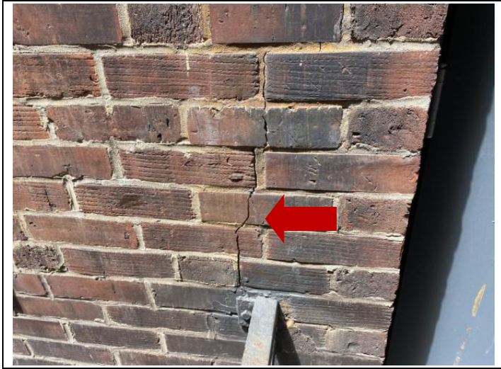
25. Cracking observed on Building B exterior wall.
