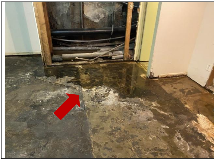
49. Standing water observed in the basement of Building D.
