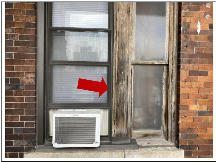
55. Typical decayed wooden window frame with several points for potential moisture intrusion.
