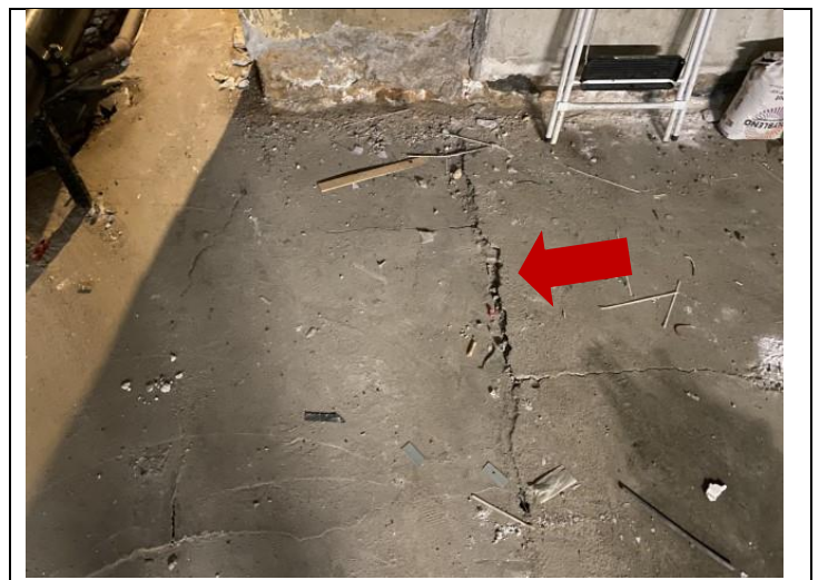
48. Cracking observed in Building D basement concrete slab.
