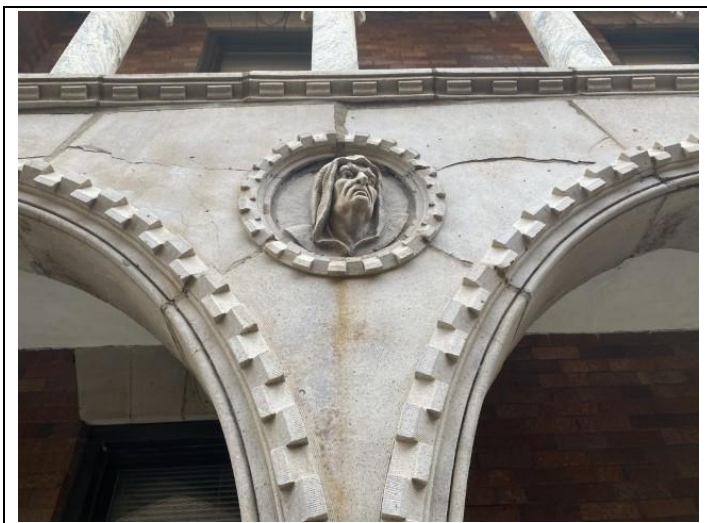
33. Typical cracking in decorative stonework in the east courtyard.
