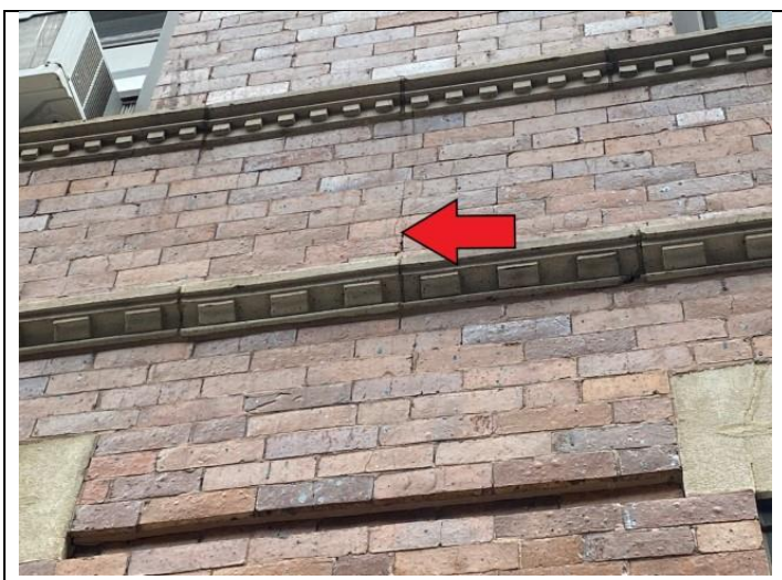
59. Typical vertical cracking in brick spandrels.
