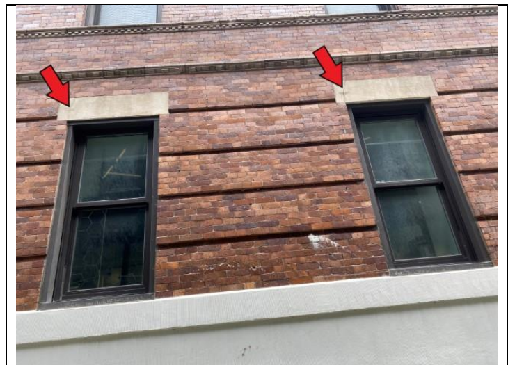
58. Typical cracks in window lintels with previous epoxy injection repair visible.
