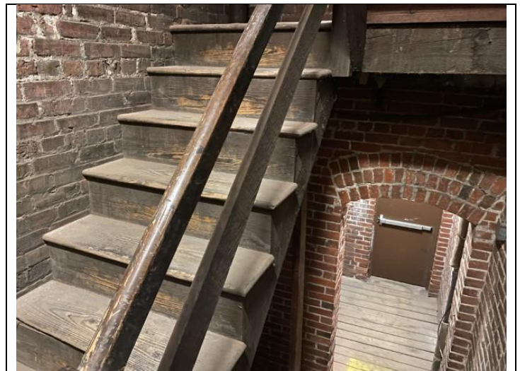
8. Typical emergency egress stairwell framing.
