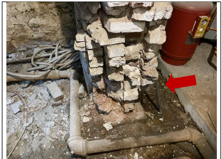
38. Distressed foundation wall with extensive spalling brick observed in Buildings G and H.
