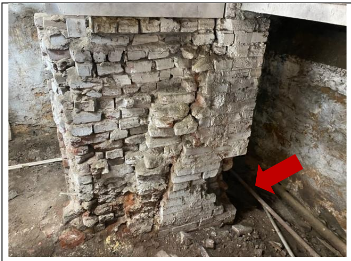
37. Distressed foundation wall with large crack on the side observed in Buildings G and H.
