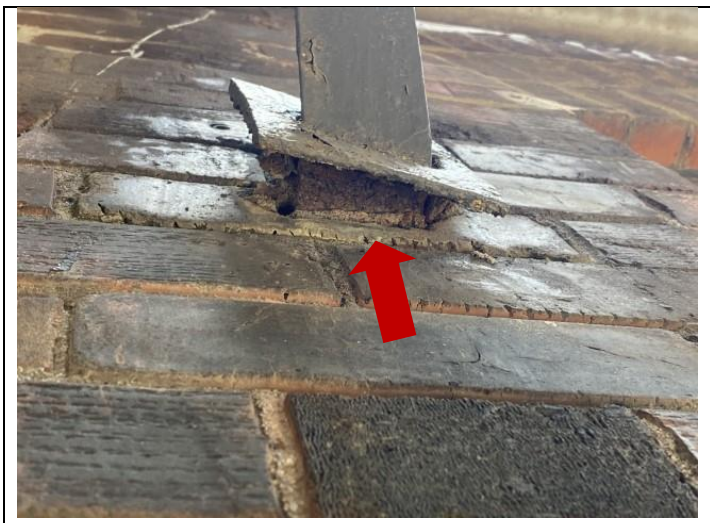
51. Typical egress balcony support separating from exterior masonry wall.
