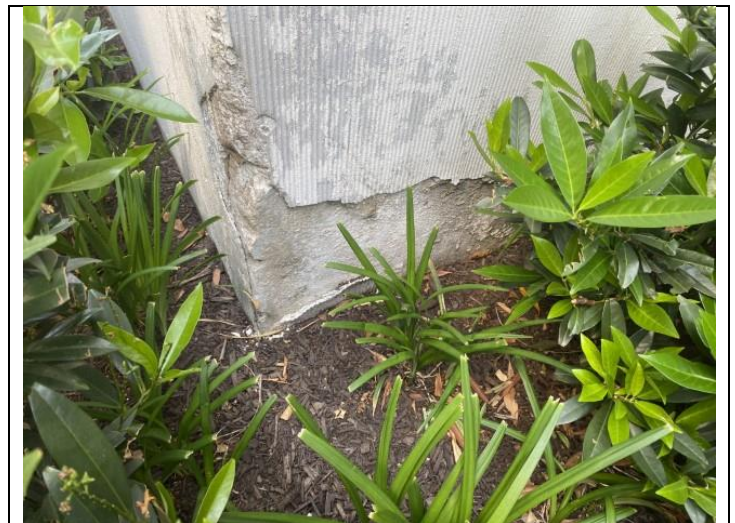
36. Spalled parging on Building A.
