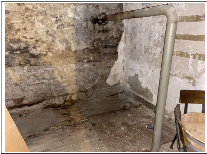
13. Exposed fieldstone foundation walls observed in the apartment buildings.
