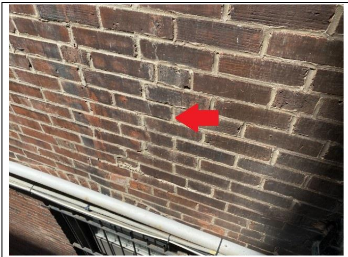
27. Additional stair-stepped cracking observed on Building B.
