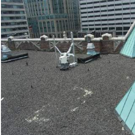
Top left, bottom left: Roof prior to replacement. Top right and bottom center: roof after replacement. Bottom right: restored bulkhead.
