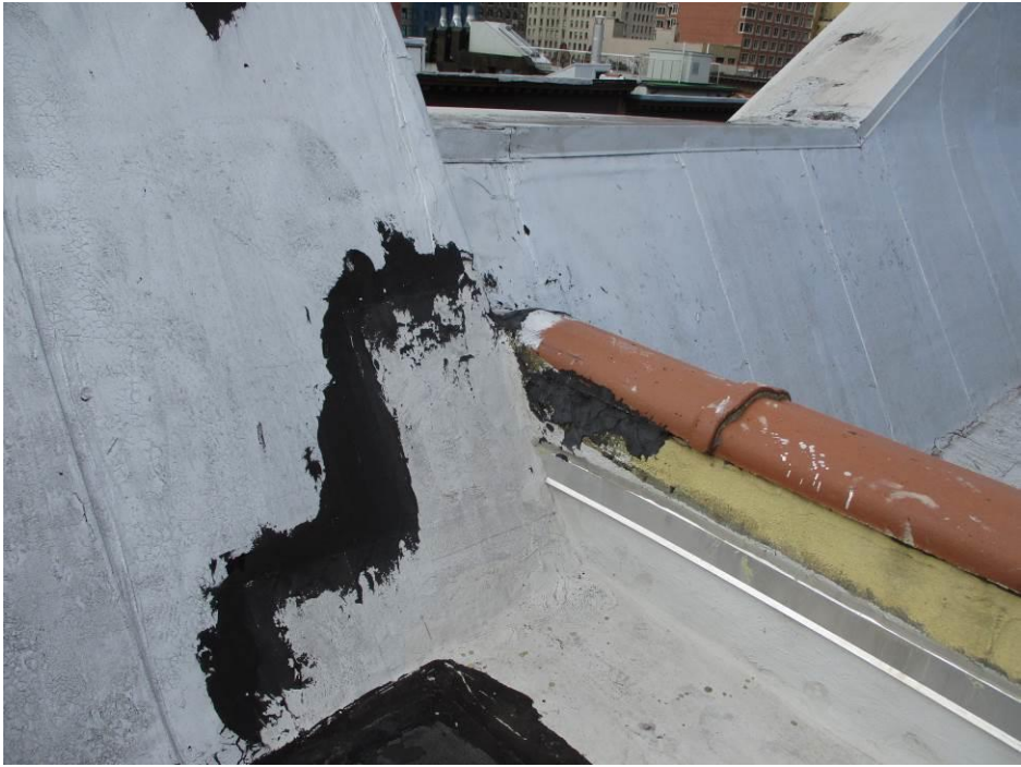
Photograph #24 Party Wall between 167 and 169 West 81 st Street, Main roof, facing South, prior to work.
