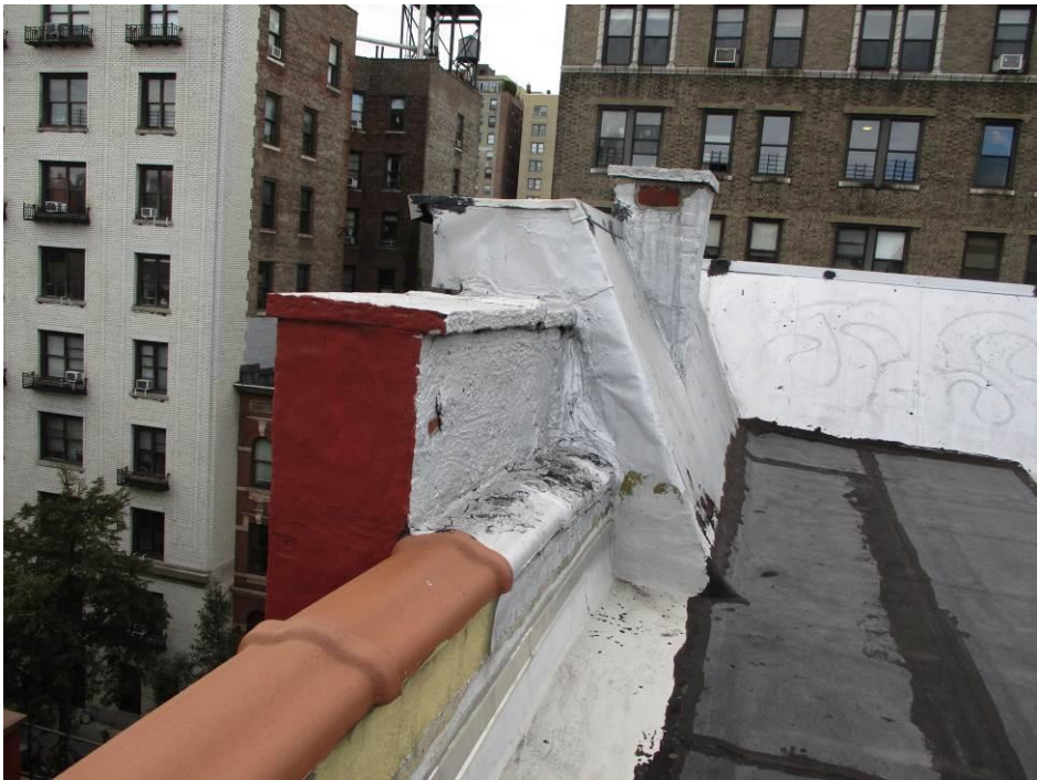
Photograph #23 Overview of 169 West 81 st Street, Main roof, facing South, prior to work.
