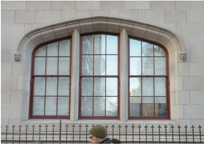
Wood window after restoration. The window restoration work encompassed thirty different window types, including arched-head double-hung wood windows, monumental leaded-glass windows set in sheet metal frames intended to imitate stone Gothic tracery, wood pivot-sash, and steel fire-rated windows.
