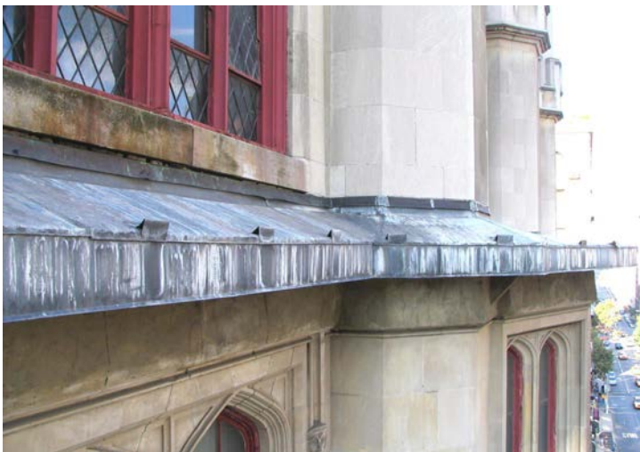
Before restoration, deteriorated metal roof and flashing over missing cornice and cracked stucco covering "scars" where original terra cotta cornice had been removed
