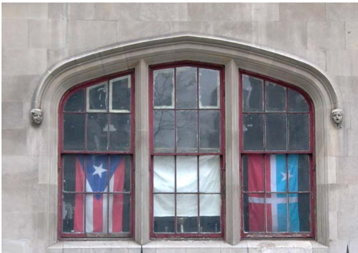
Wood window before restoration. All original wood window frames were restored by epoxy consolidation and installation of wood dutchmen, as well as the fabrication and installation of new wood sash with clear Low-E insulated glass for energy efficiency.
