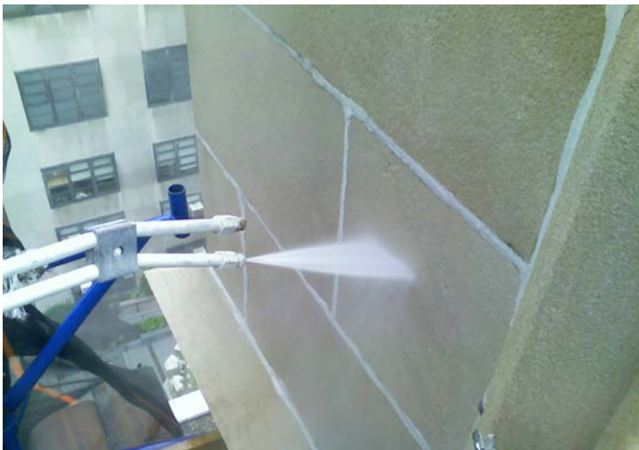
The scope of work on this restoration included a full cleaning of the building's limestone.
