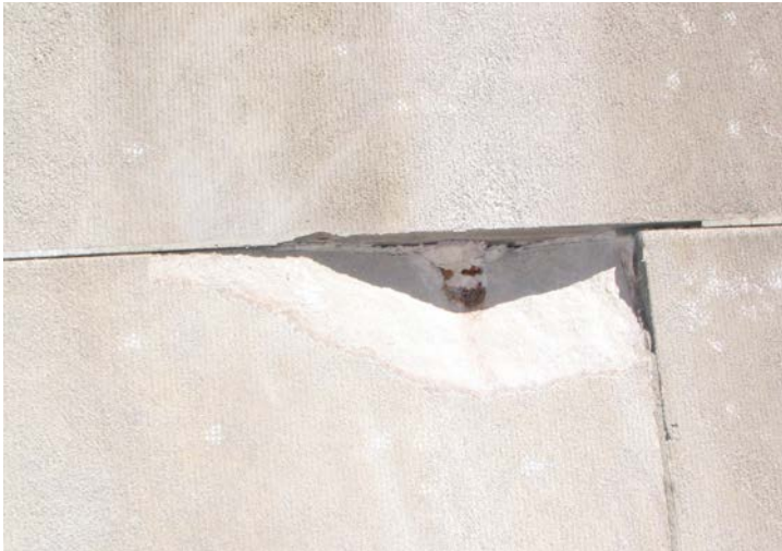
Typical existing condition: limestone deterioration at rusting iron cramp
