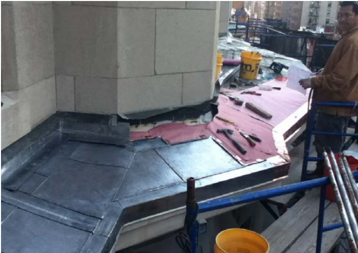
Lead coated copper roof was installed on top side of the new cornice.
