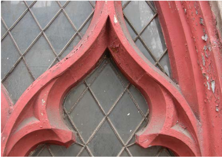
Leaded window before restoration.
