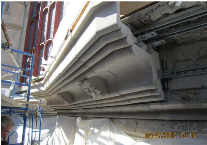
Reconstructing cornice -- underside done with glass fiber reinforced concrete. Photo research was conducted to reproduce design of original terra cotta cornice.
