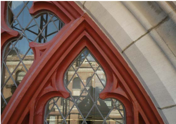
Leaded window after restoration. For the leaded glass windows, work included restoration of rusted sheet metal frames with sheet metal and epoxy patches, reglazing of zinc-leaded panels with new lead comes and new clear glass, restoration of steel pivot sash, reinstallation of re-leaded panels.
